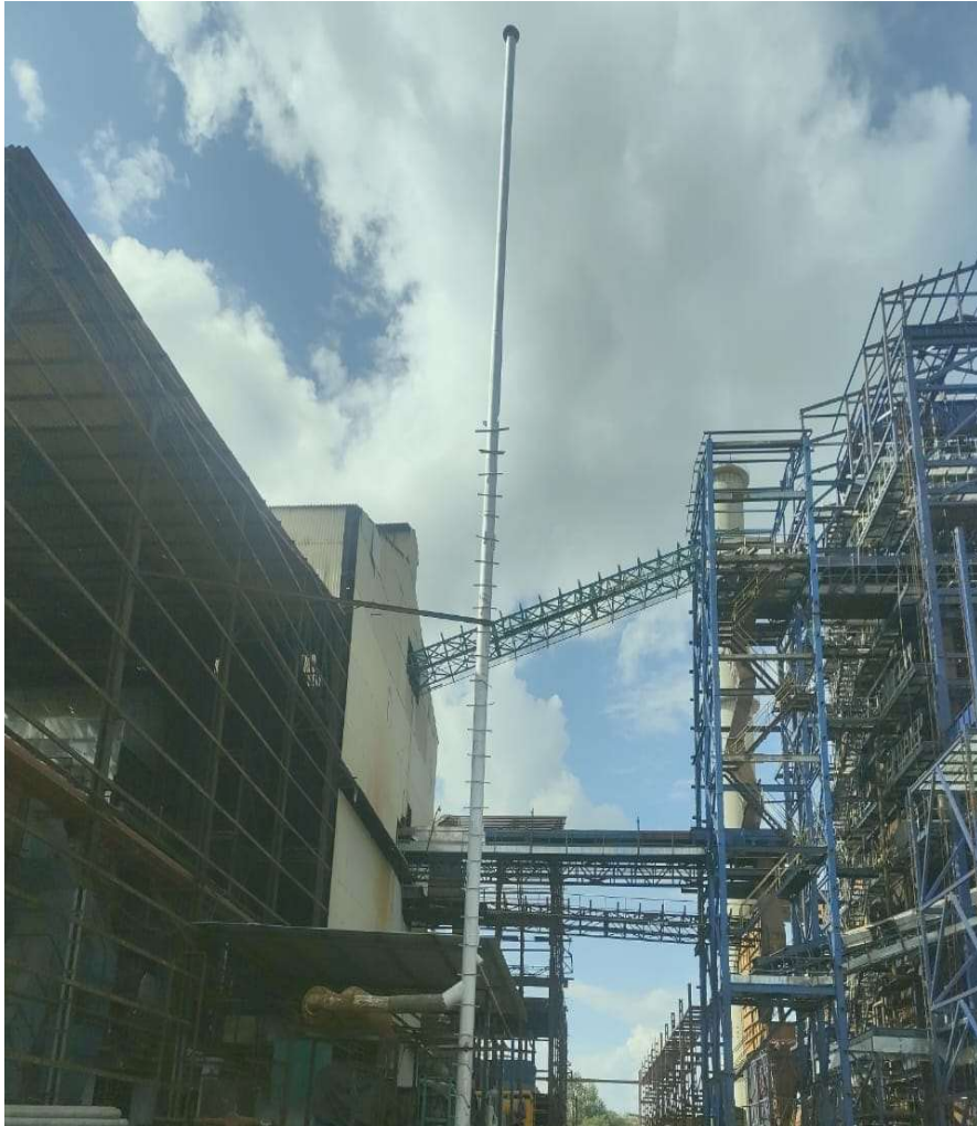
PHOTOGRAPH OF DG SET WITH CHIMNEY (30 mtr. HEIGHT)
